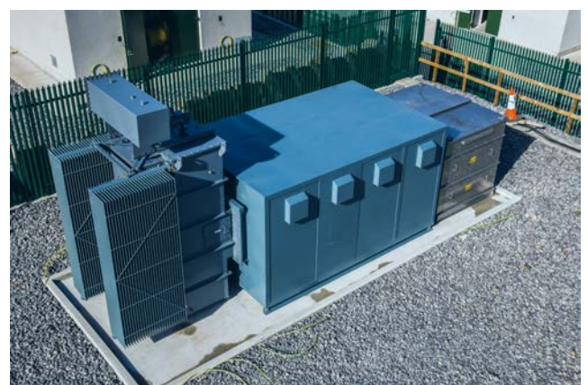
Figure 2 - Enspec C-type Harmonic Filter
